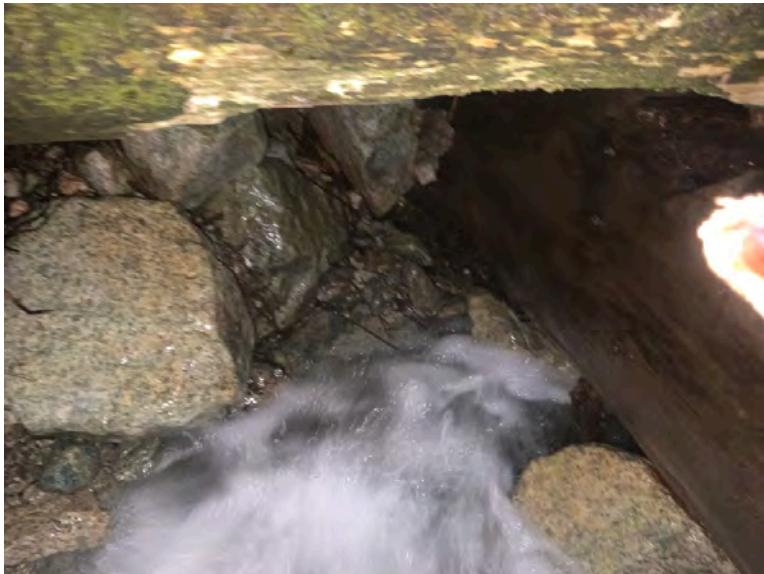
Inlet erosion behind sill log upstream left side
